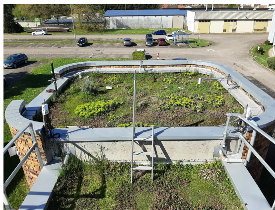
Figure 2: Green roof located in the Cerema of Tomblaine, close to Nancy, France.
